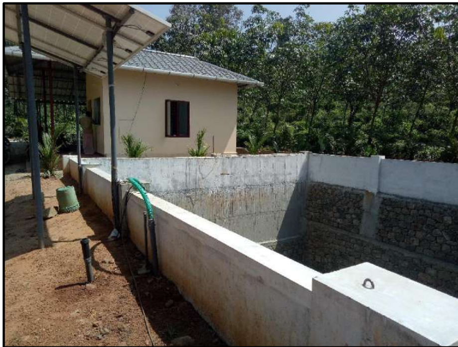
Photograph showing the rain water harvesting tank
